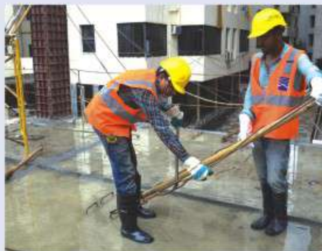
PPE (helmet, hand gloves, gum boot and safety vest) worn by workers while doing column shuttering work at Sheltech MRC Garden
