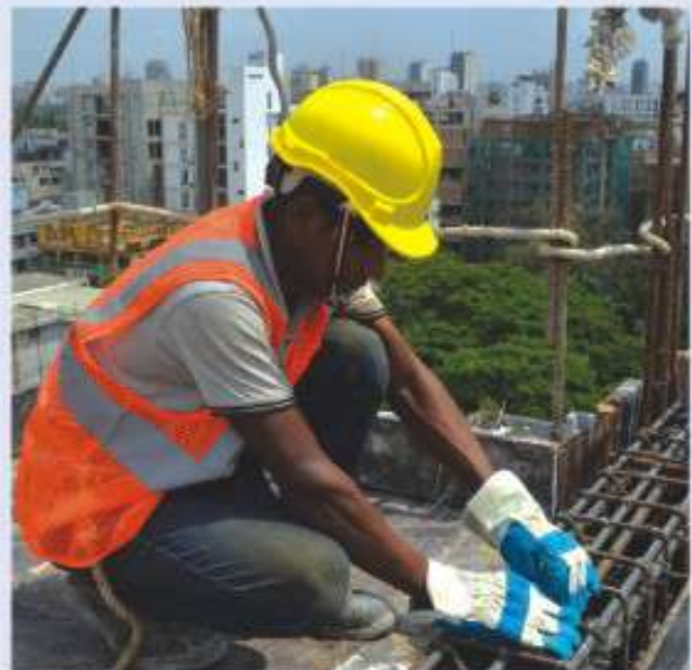
PPE (helmet, hand gloves, safety vest, safety belt and safety shoes) worn by worker while binding reinforcement at Sheltech Ayaan at Banani 11
